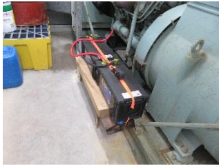
Batteries needing replacing
