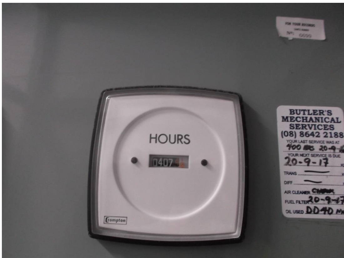
Engine Hour Run Meter
