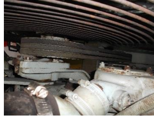
Fanbelts needing replacing
