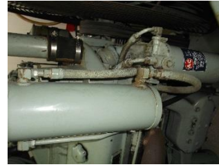
Fuel pipes needing replacing
